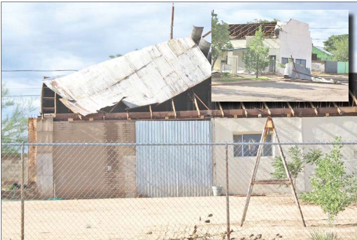
Strong winds ripped off the roof from this warehouse.
